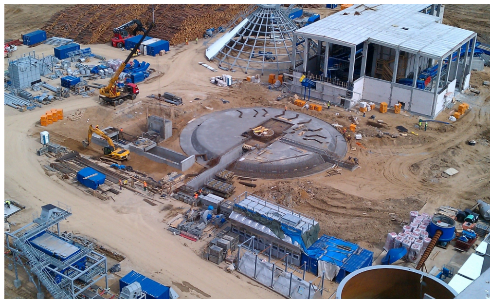
silo base plate and debarker - / chopper building
