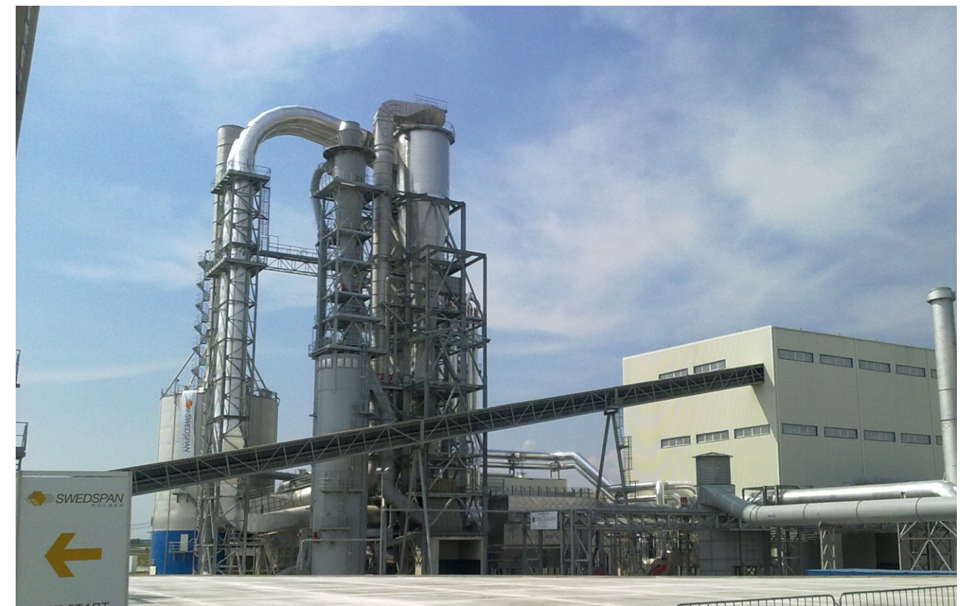
photo refiner building, dryer cyclones
